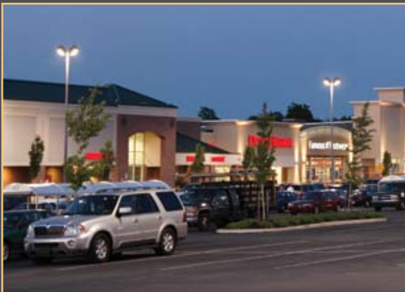
Site and Area Lighting
